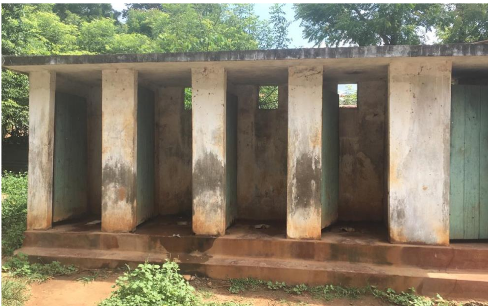
A public toilet at an IDP camp in Tellippalai, Jaffna
